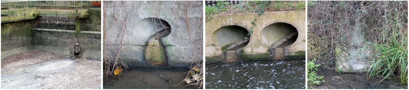
Ewell Storm Tanks
